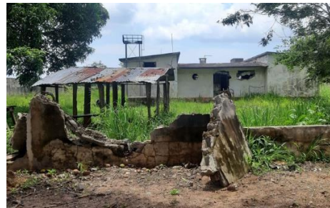
Photo 2: Destruction of the prison of Mocímboa da Praia
